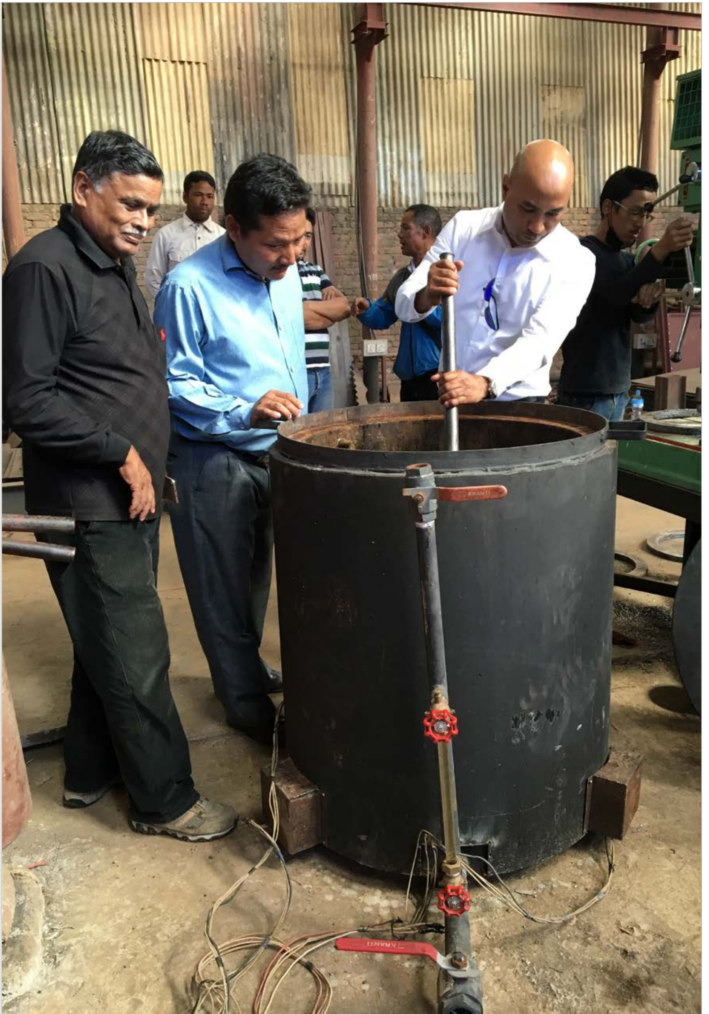
Photo: ITC, New technology for electric boiler, HANDPASS and AEPC project
